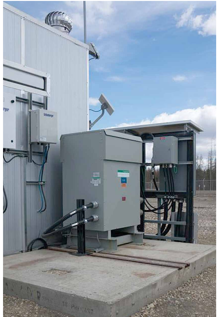
The SCB3 transmits real-time data via satellite from remote wellsites located almost anywhere in the world.
