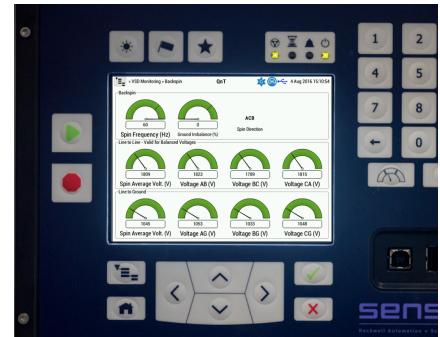
Live High-Voltage Measurements
