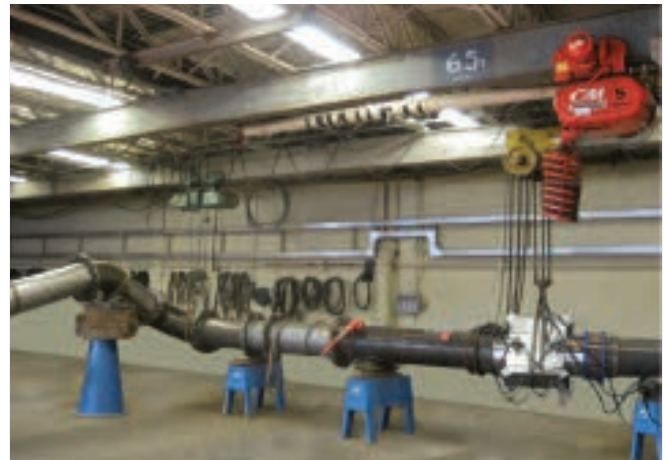
LEFM metering spool installed downstream of several out-of-plane elbows
