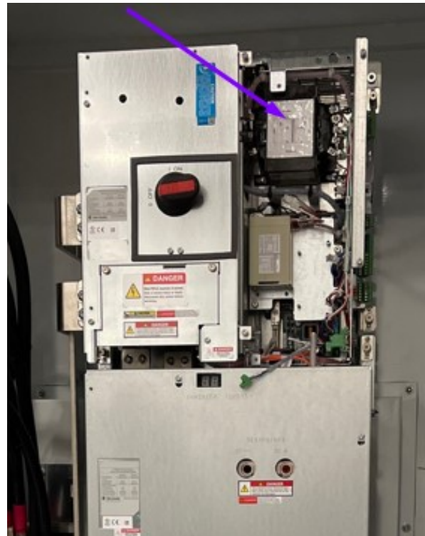
Figure 5-17: Location of CPT in a DC-input drive (top right corner)
