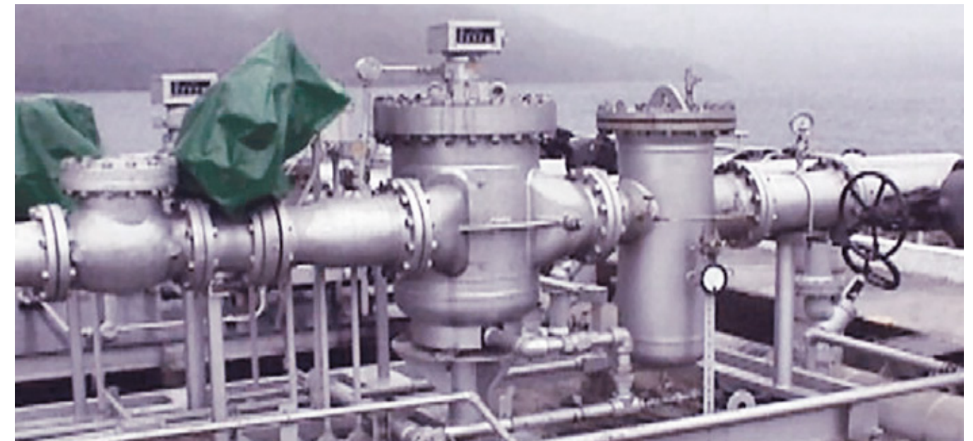
Fuel oil bunker blender
