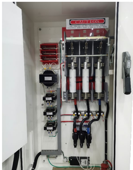
Figure 1.3: INSTRUCT ESP Switchboard High Voltage Compartment
